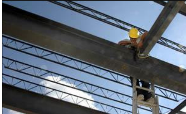
Photo by Joe Imel/Daily News Charles Strode of Tompkinsville, an employee of The 31 Corp., connects beams Monday at the site of the new Bowling Green Area Chamber of Commerce building at College Street and Seventh Avenue. Houchens Industries has contributed $400,000 to the project and has earned naming rights. The building will include the title Houchens Industries Center for
