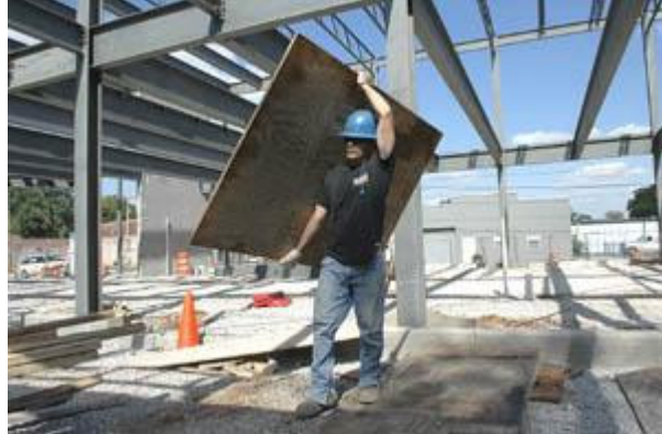
Photo by Joe Imel/Daily News Scott & Murphy's Bruce Williams, of Rock Creek in Grayson County, carries wood Monday across construction site of the new Bowling Green Area Chamber of Commerce building at College Street and Seventh Avenue. A basement added to the final design of the building for storage has brought the two-story structure to 17,500 square feet, an increase from the 15,000 square feet.
